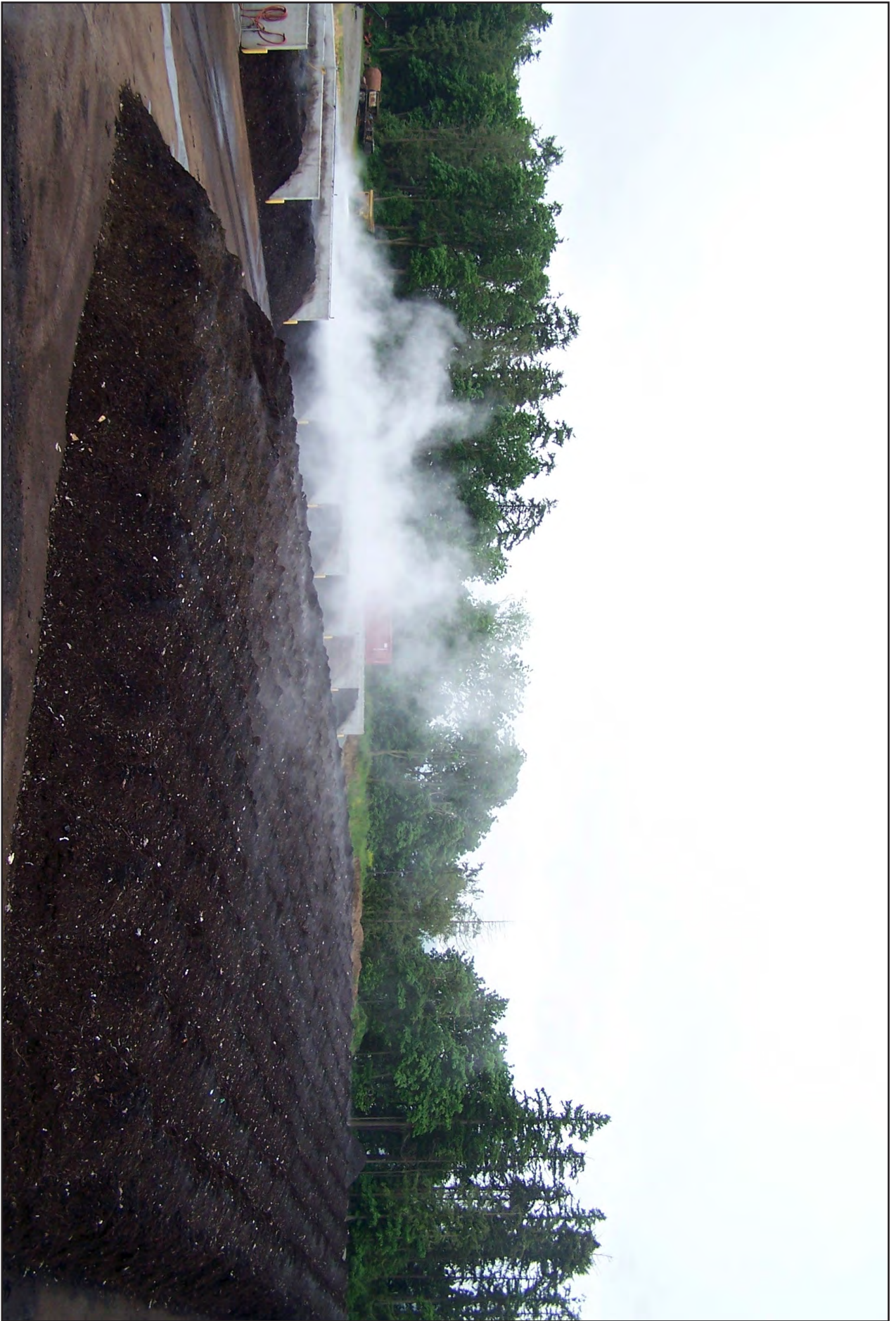
Activity 3 - 4023 - Facility overview, 2011. Washington. (Lenz Enterprises, Inc.)
