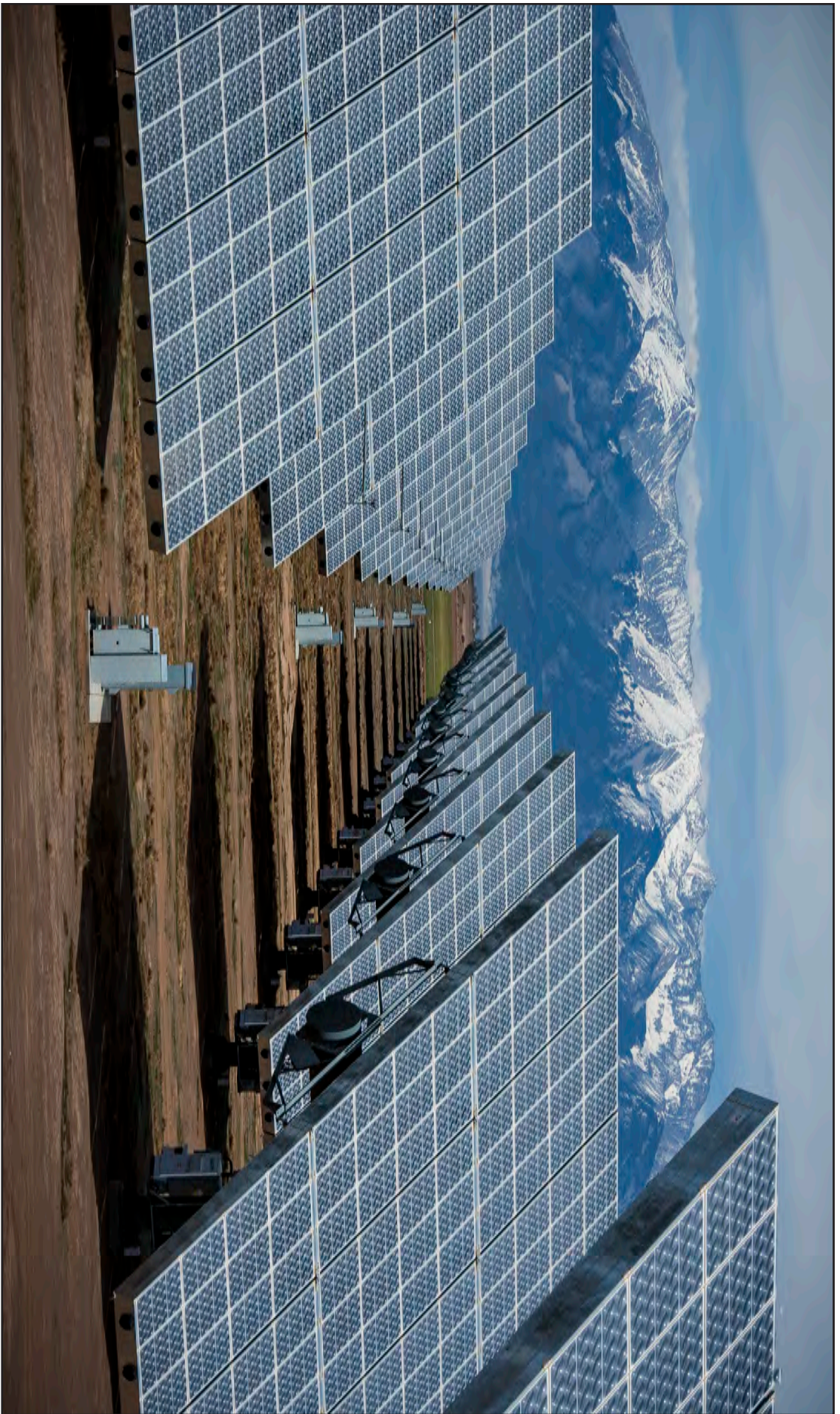
Activity 2 - 2598 - Alamosa Solar Generating Project is the largest high concentrating solar photovoltaic power generation system in the world. Alamosa Solar consists of over 500 dual-axis, pedestal mounted tracker assemblies, each producing 60 kW. Each tracker assembly is 70 ft. wide by 50 ft. high and contains 7,560 Fresnel lenses that concentrate sunlight by a multiple of 500 onto multi-junction cells. The photovoltaic assemblies were provided by Amonix Alamosa Solar and is located on 225 acres in the San Luis Valley near Alamosa, Colorado. May 5, 2014. (Dennis Schroeder/NREL 31439)
